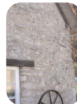
Inappropriate hard cement mortar
