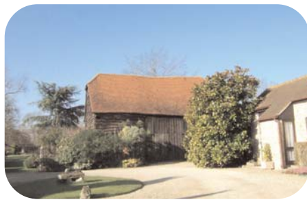
Half-hipped clay tile roof and weather- board, barn NW of Westfield House
